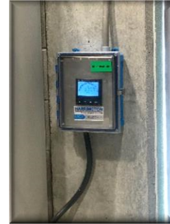
Figure 19: Ozone Analyzer (Return from Tank) 337mV. COMMENT: Consider reducing ozone dosage to drop ORP in tank as low as possible. Modify system operation to accommodate algae growth.
