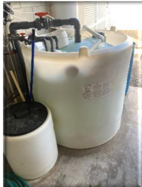
Figure 26: Chlorine Storage COMMENT: Ozone being added with addition of manatees.
