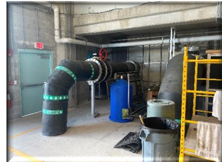
Figure 16: LSS Piping at Degas Towers
