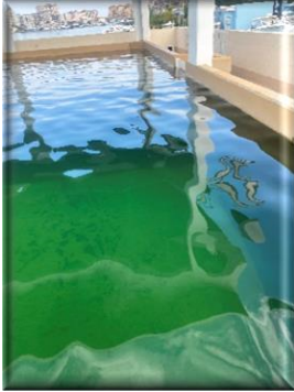
Figure 22: Rescue Deck Pool COMMENT: Direct sunlight requires chlorination and scrubbing to control algae.
