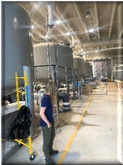
Figure 14: Main Filters. COMMENTS: Mechanical Seals Leaking. Use of Defender Filters and Fractionators to allow for fish at heavy loading.
