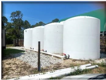
Figure 30 Stranding Center Storage Tanks
