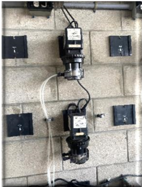
Figure 25: Rescue Deck Pool Chlorine Feed Pumps
